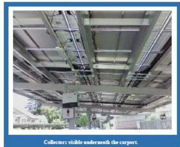
Collectors visible underneath the carport.
