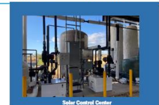
Solar Control Center
